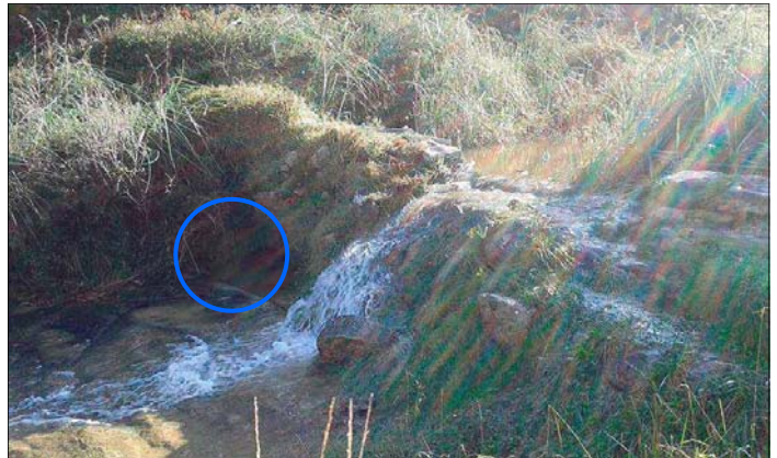
Sluice gate installed and closed to evaluate its performance. The water does not run through the base outlet (blue circle), but flows over the small dyke.
