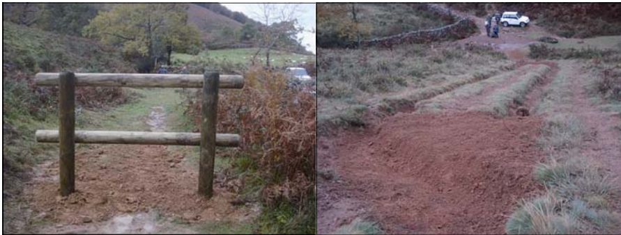
From left to right: Barrier to prevent vehicles from passing. Crosswise drainage to divert torrent water to the track drainage system.
