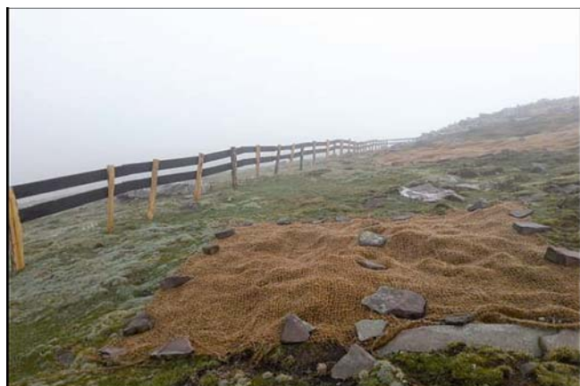
Xuriain Mire: Natural-fibre mesh protecting eroded areas at the Xuriain site. The mesh is secured with corrugated steel rods and local stones.
