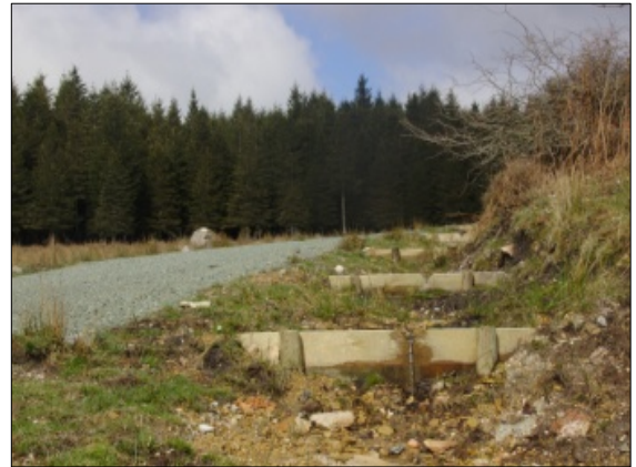
Dykes to check the water in the ditch of the Usabelartza track.
