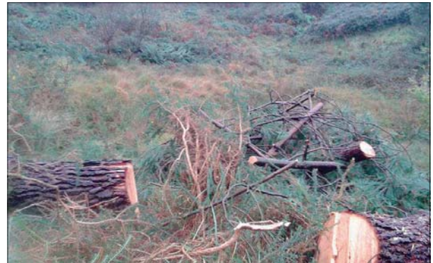
Forestry debris removal in progress (unchopped debris), with part of the wetland in the background.
